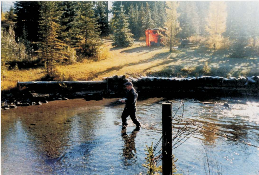
Photo V-6 Log Crib Wall Retaining the Right Downstream Bank of Policeman Creek in the Vicinity of a Private Residence (not part of Restwell property)
